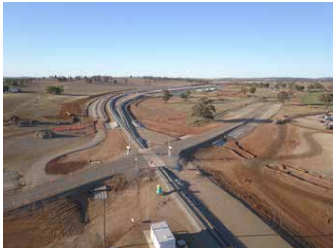
Work is complete on the North West Connection, which joins Inland Rail to the existing Broken Hill track.
