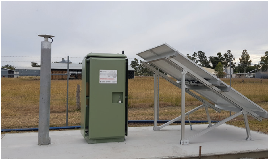
CORS installed at Cecil Plains in support of the Inland Rail program.
