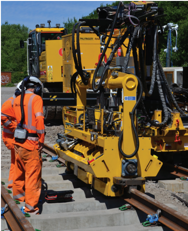
Inland Rail will be able to utilise induction welding once testing is completed and proven to be compliant with ARTC standards.
