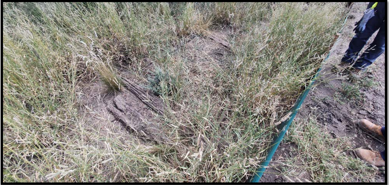
Plate 5-5. Temporary habitat enhancement works in Stage 3 using timber and hay biscuits to increase ground cover for relocated FCWS.
