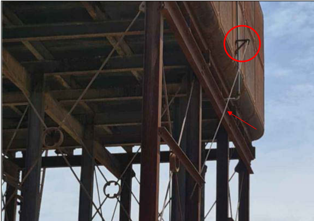
Figure 1-3: Close up image of the wire (arrows) and bracket (circle) proposed for removal.
