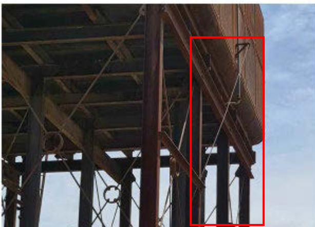
FIGURE 2.5 MILVALE YARD WATER TANK WITH WIRE ENCROACHMENT (SEE RED OUTLINE)
