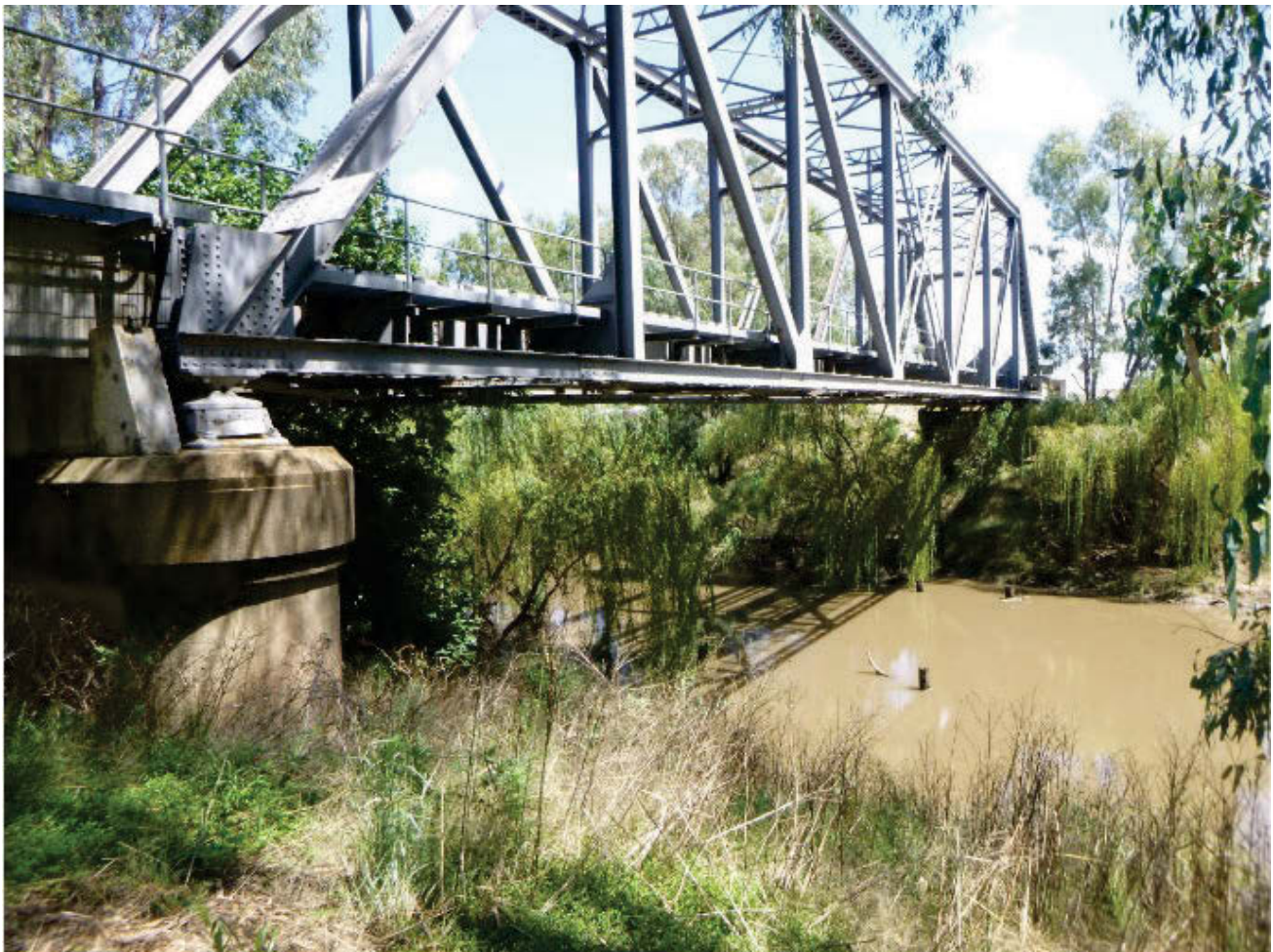
FIGURE 5.2 VIEW FROM THE NORTHERN BANK OF THE TIMBER PIERS IN THE RIVER IN RELATION TO THE BRIDGE
