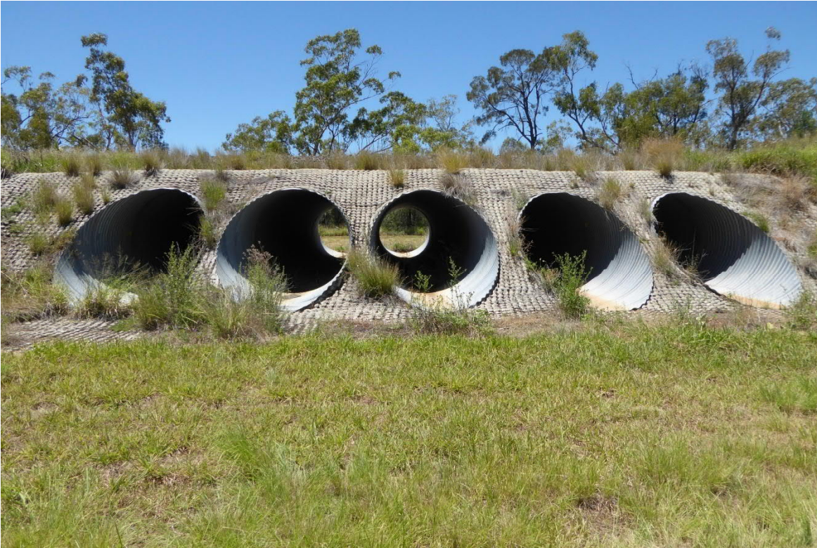
Figure 4.4 Photos of example culverts showing typical level of blockage – 621.848km
