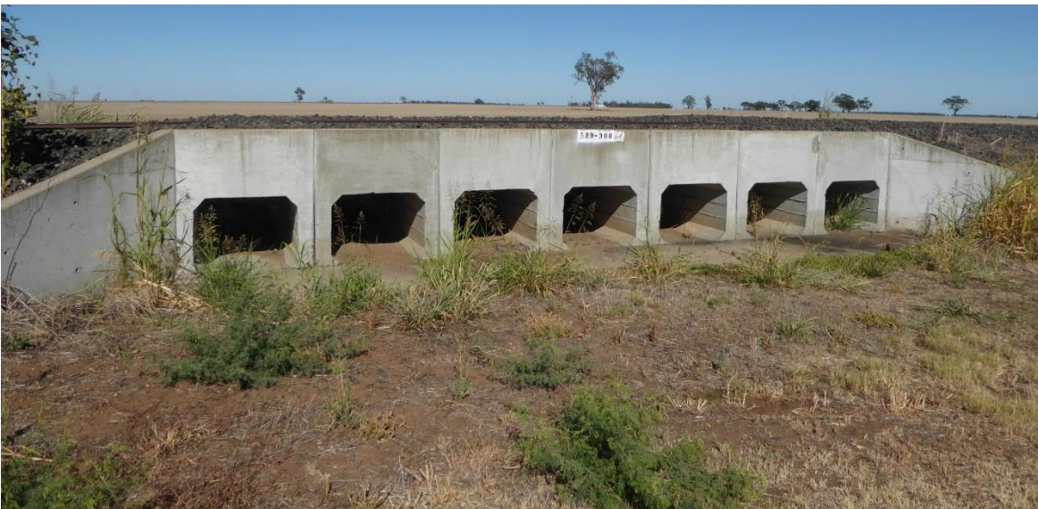
Figure 4.3 Photos of example culverts showing typical level of blockage – 589.3km
