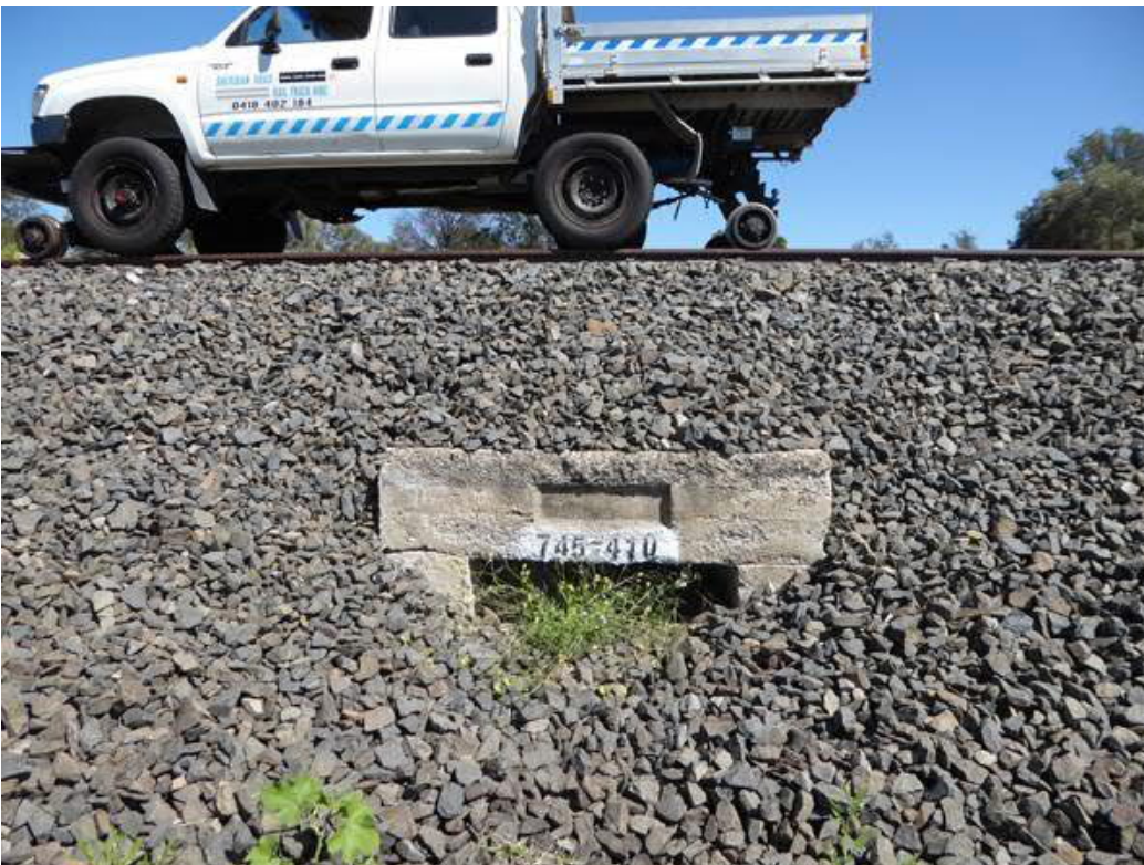
Figure 4.5 Photos of example culverts showing typical level of blockage – 745.41km
