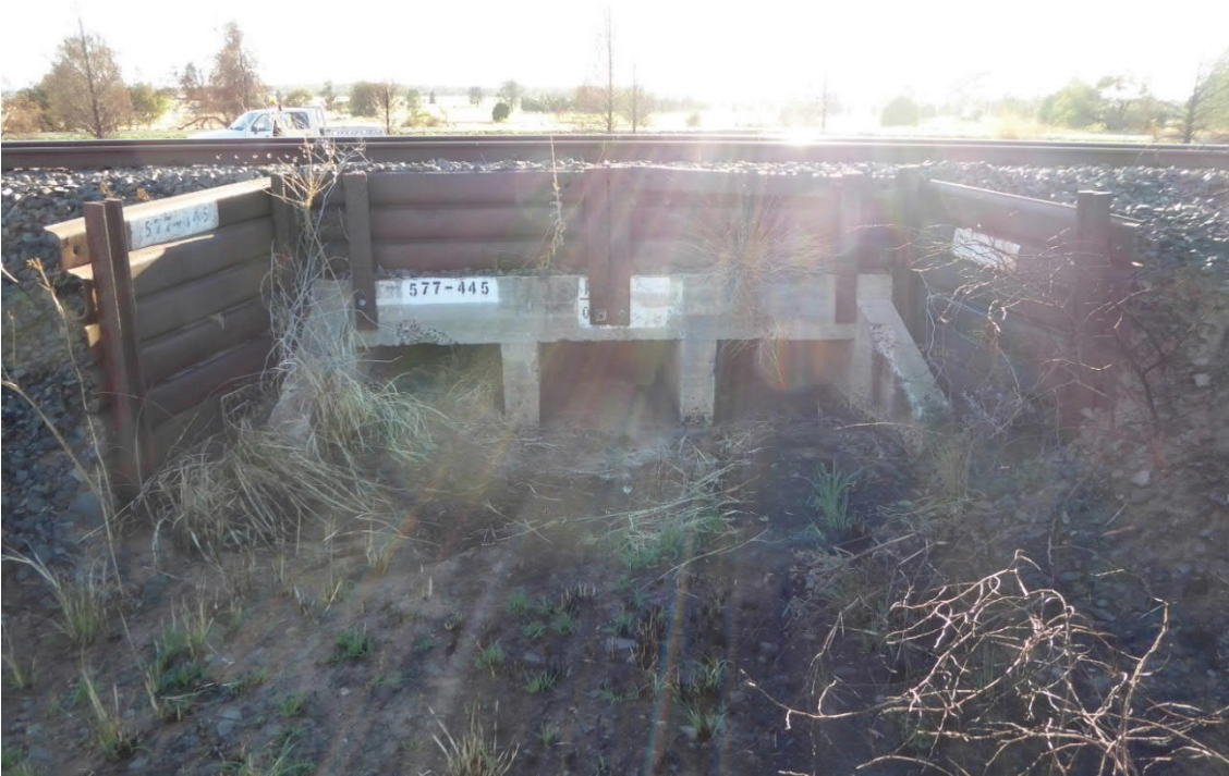
Figure 4.2 Photos of example culverts showing typical level of blockage – 577.445km
