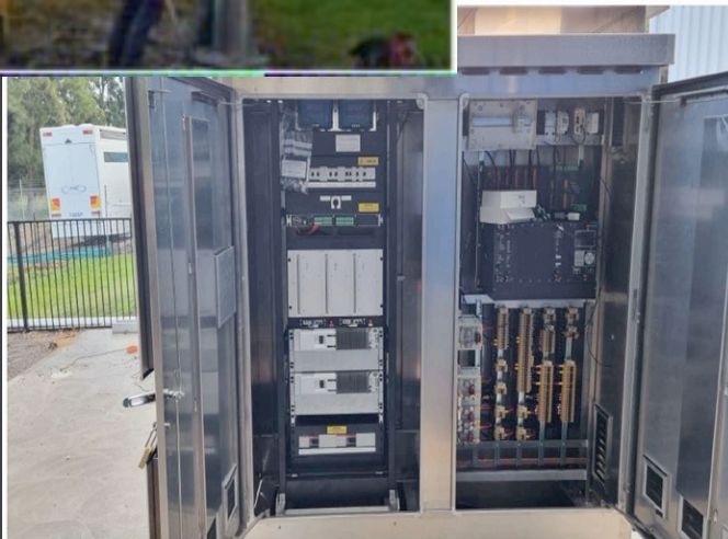
Solar Powered Location Case interna (Sentinel Power Rack on left, GCP on Right)
