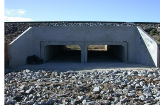
Erosion and scour rock protection at culvert outlets
