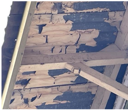
Figure 3-10: Deterioration of protective coating system on roof sheeting
