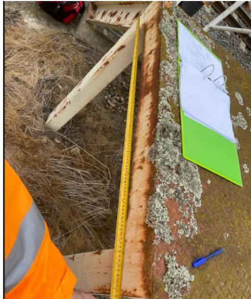
Figure 3-14: General surface corrosion on one of the PFC members of the external staircase
