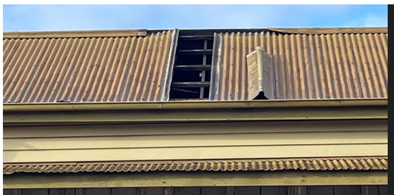
Figure 3-8: Section of roof sheeting missing and section of the roof ridge on top of the roof
