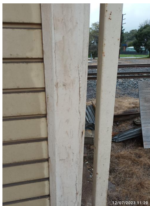
Figure 3-17: General photo of main column on the south-east corner of the building
