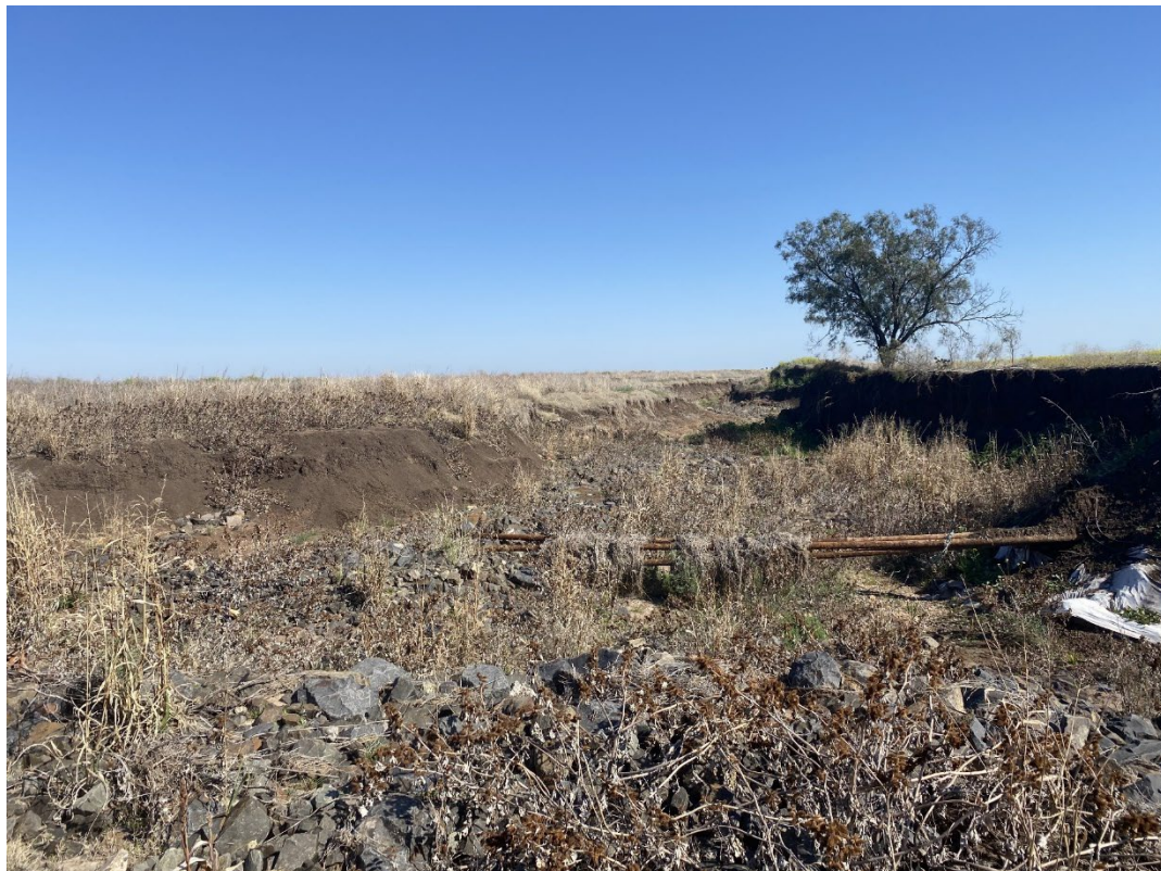
Plate 28 – Erosion at Boggy Creek from high-velocity flows during 2022 floods (operational)
