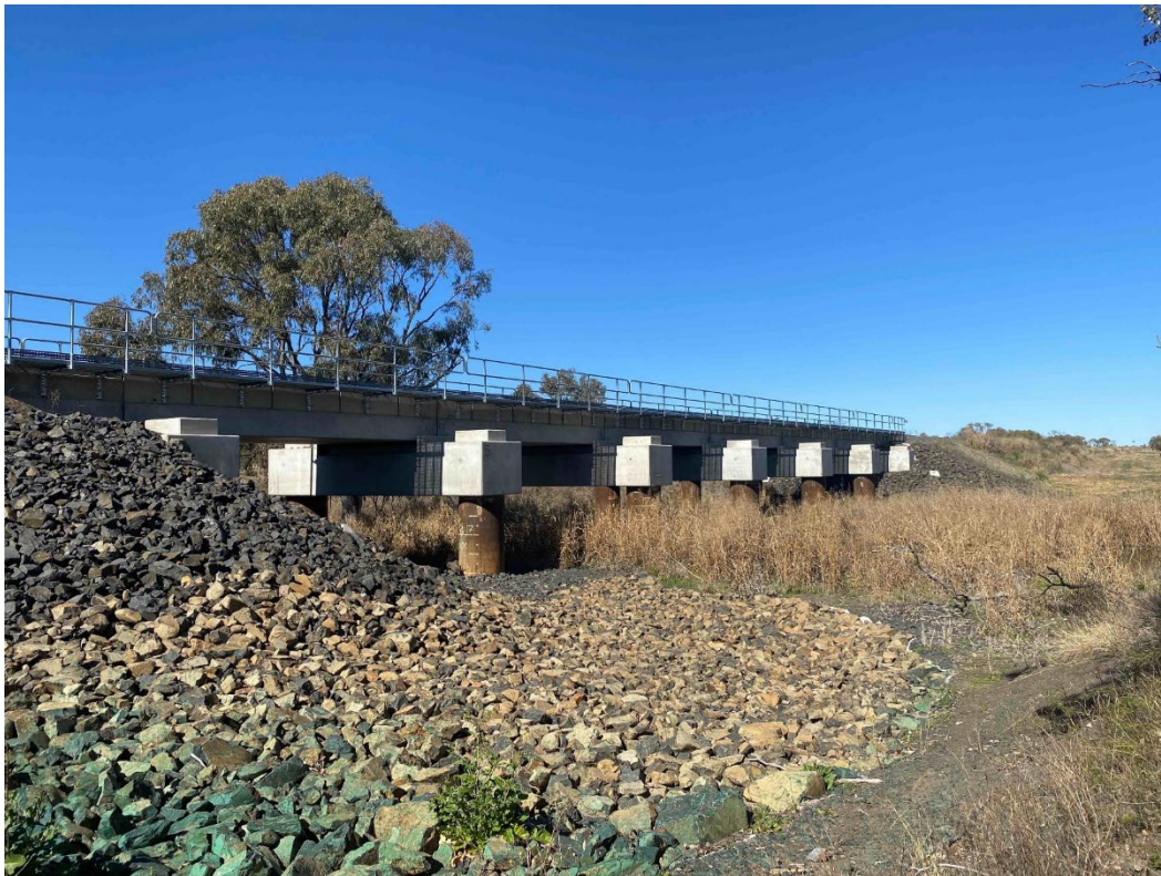
Plate 10 – Yallaroi Creek Bridge with heavy weed presence
