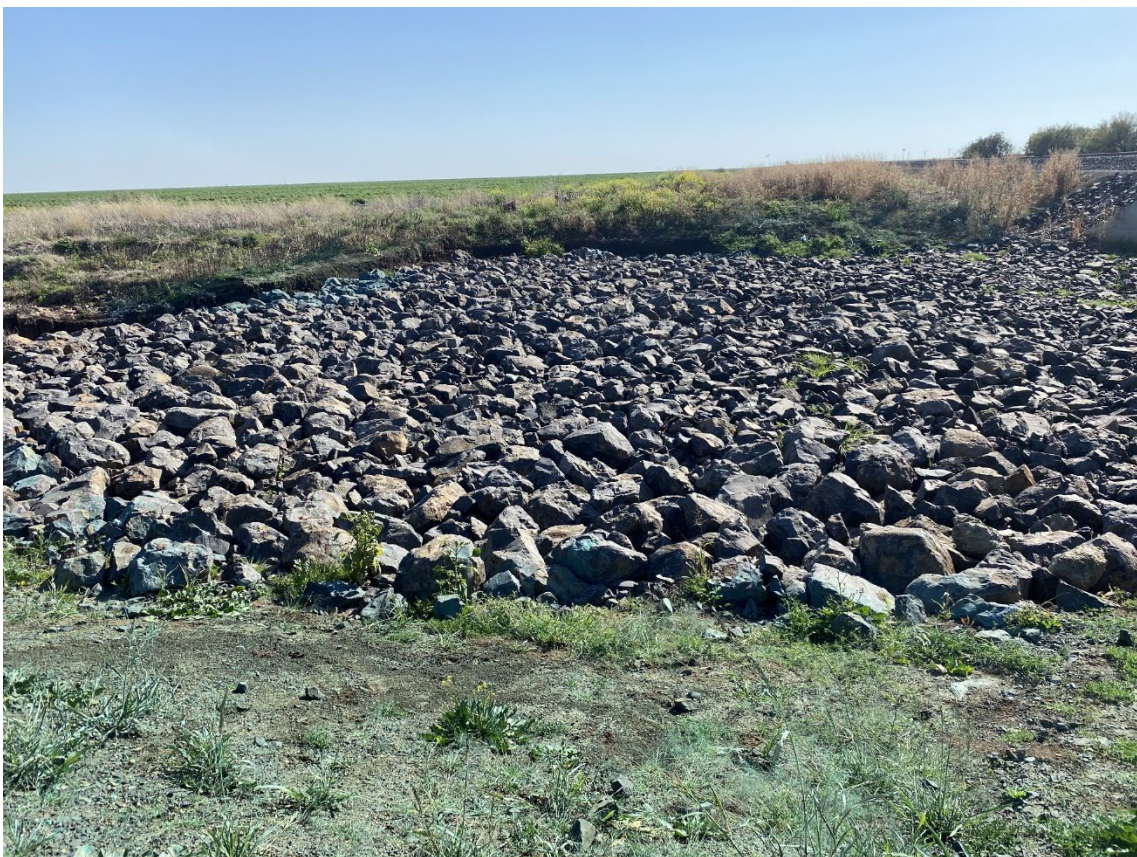
Plate 24 – New flood design rectification works after heavy flooding during Audit 4, including heavier rock armouring and hydromulching along batters at Bulldog Creek (operational)
