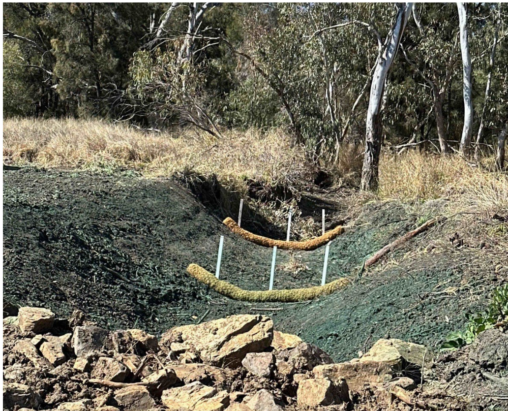
Plate 12 – CH744 Culvert 566 ERSED controls including coir logs and hydromulch where vegetation has not yet grown
