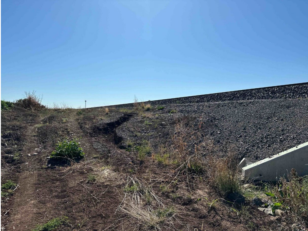
Plate 29 – Eroding longitudinal drains at Boggy Creek (operational)
