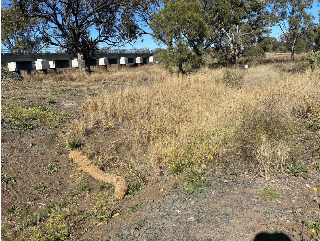
Plate 11 – ERSED controls in place in areas of limited vegetation cover at Yallaroi Creek
