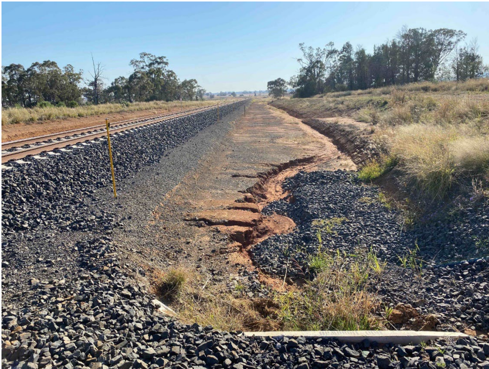
Plate 18 – Severe erosion, no vegetation cover or ERSED controls at LX3056 (operational)
