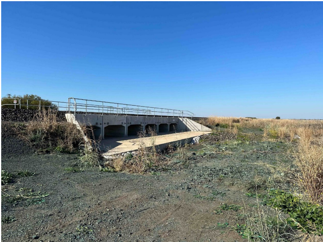
Plate 22 – Pan Creek Culvert with heavy flood damage (operational)
