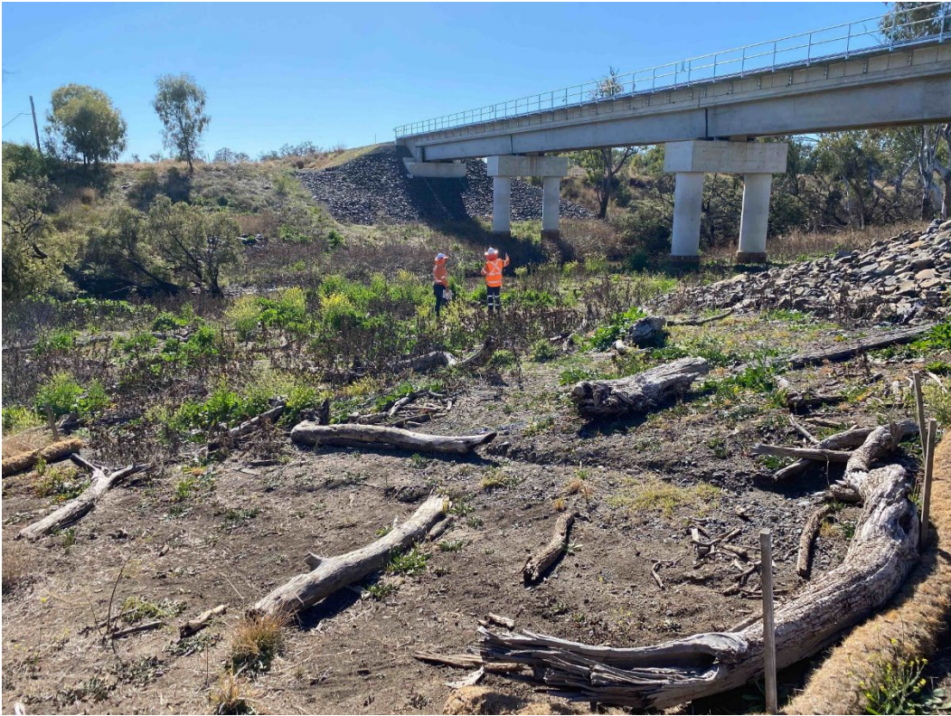
Plate 7 – Croppa Creek Bridge with high levels of weeds with habitat logs and ERSED controls present
