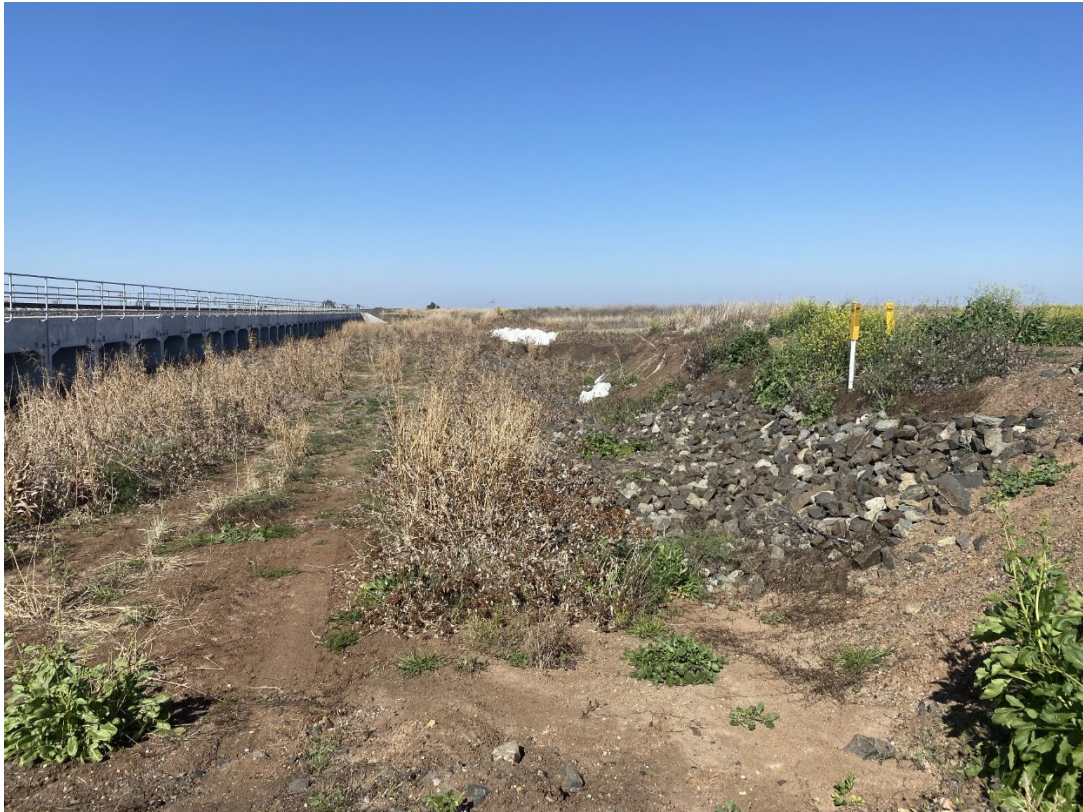
Plate 27 – Scouring from severe flood event in late 2022 at Boggy Creek (operational)
