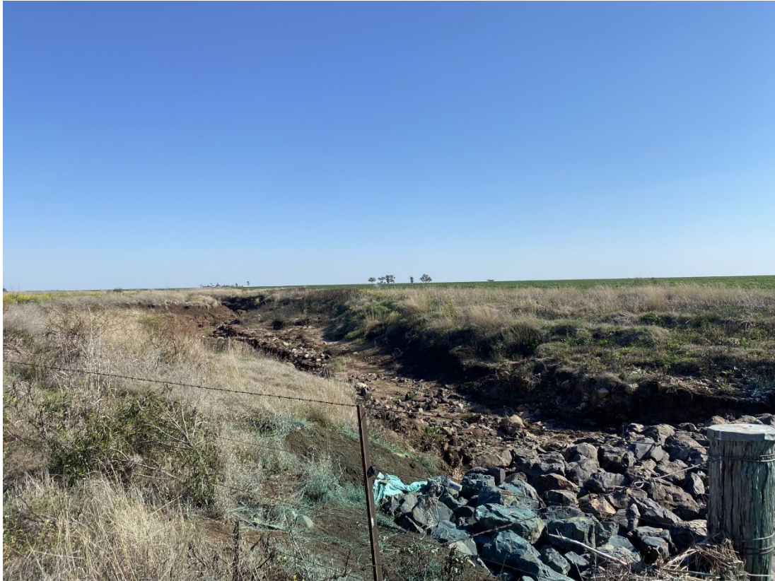
Plate 25 – Eroded creek bed downstream of Bulldog Creek from flooding (operational)
