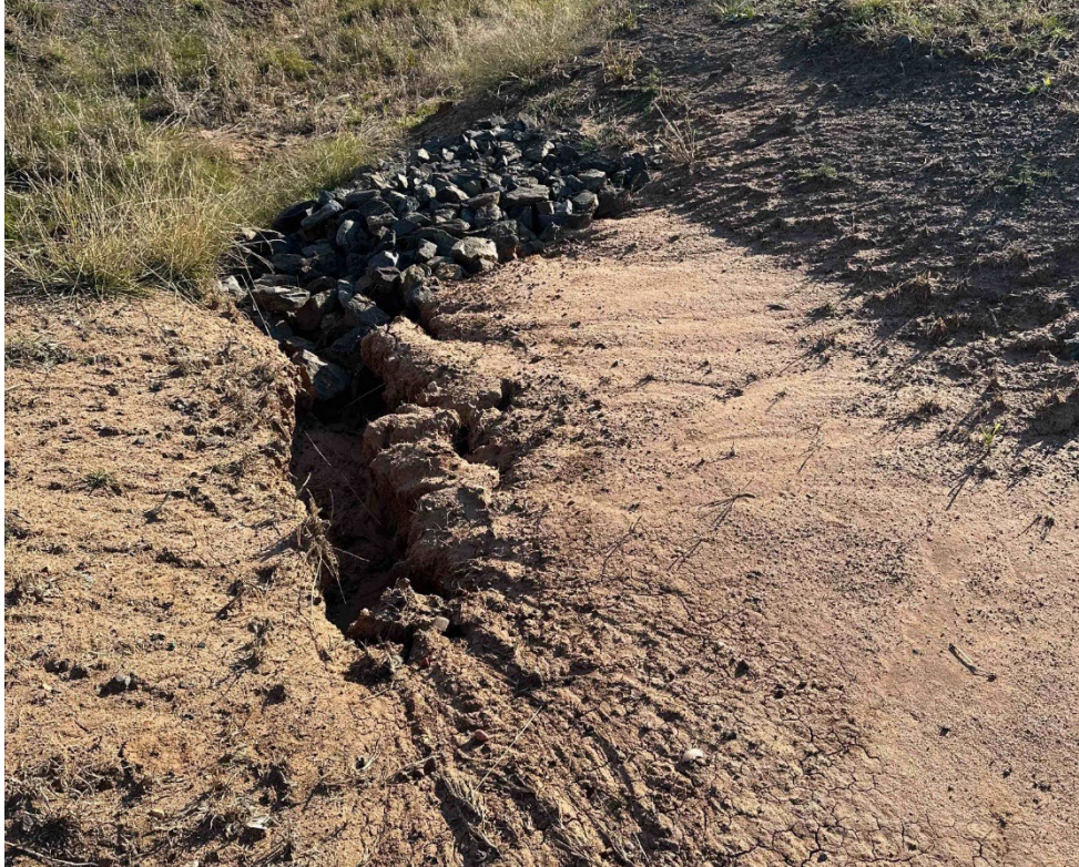
Plate 17 – Major rilling and erosion at Gate 2 longitudinal drain (operational)
