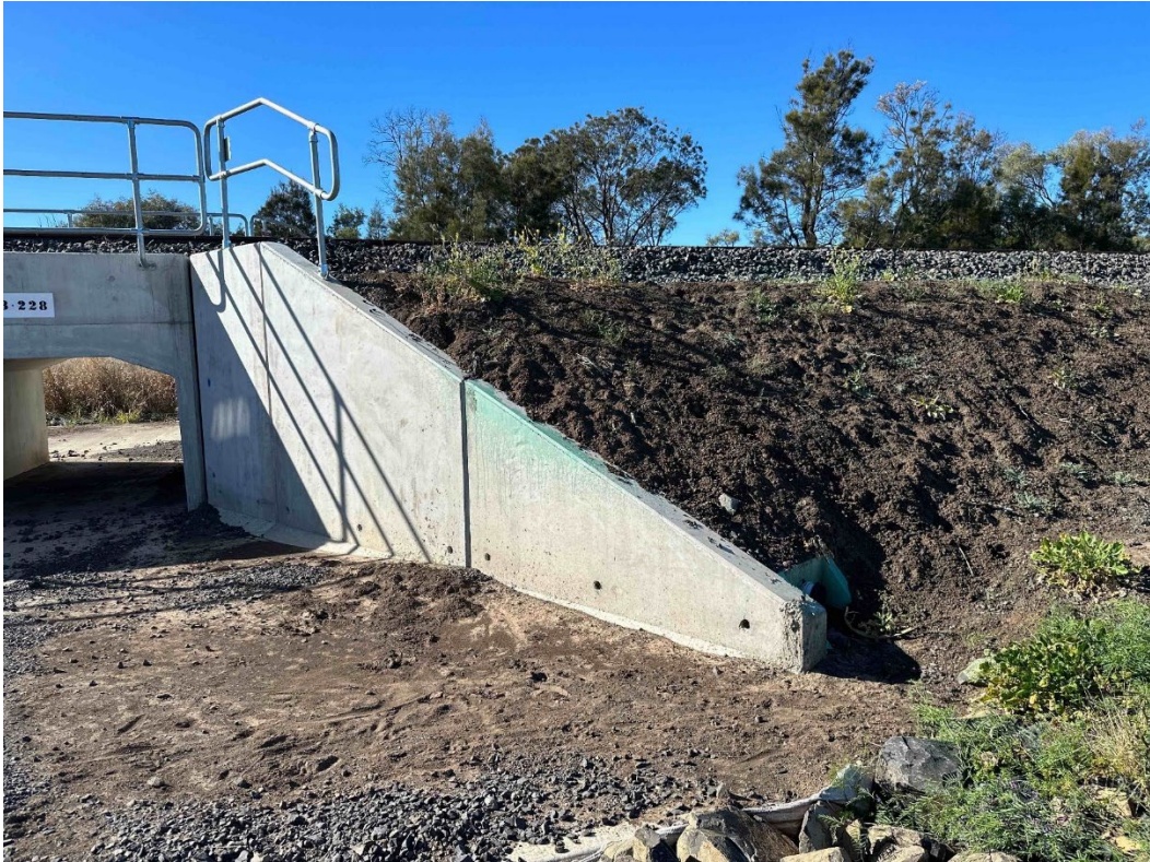
Plate 5 – CH723 Culvert 228 with limited vegetation cover and low level rilling
