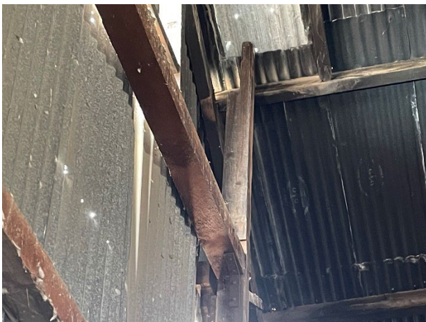
Photo 3: Previous column lean at Upend wall
