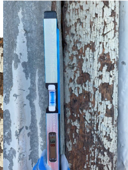
Photo 2: Current incline at Downside wall (Jan 2024)
