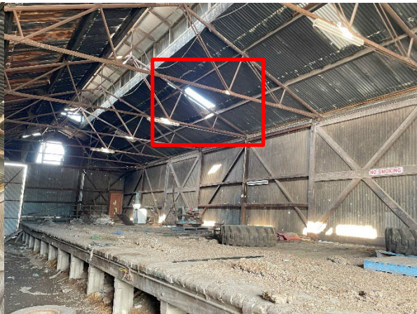
Photo 6: Current steel roof sheet missing
