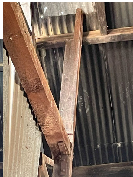
Photo 4: Current column lean at Upend wall
