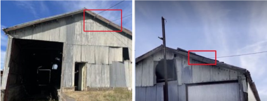
Photos 10A&10B, location of power lines connected to the northern and southern ends of The Shed (left to right)
