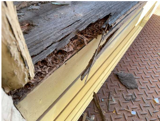
Photo 4: Upstairs Step rotting
