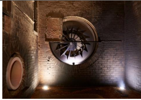
Figure 19: Industrial fan at the Burnley Maltings was repurposed to create a sculptural table. Source: Hin Lim Photography.
