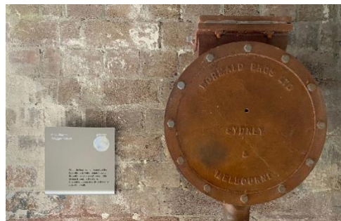
Figure 18: Signage at Substation 164 by Trigger and GBA Heritage. Source: Trigger and Built.
