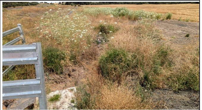
North of Boonery Park Rd - LX3165 area of scour within Pearlman Property.
