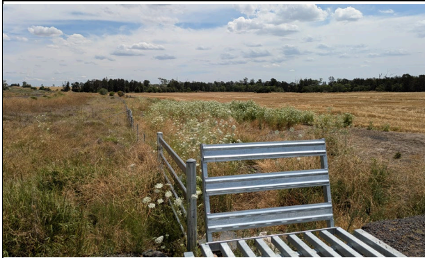
North of Boonery Park Rd -LX3165 area of scour within Pearlman Property.
