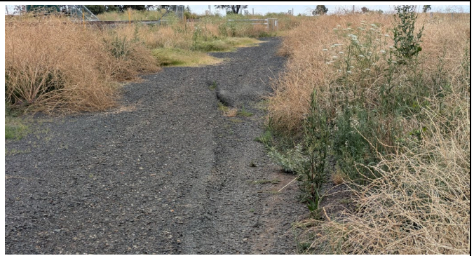
North of Boonery Park Rd – View north at LX316 showing erosion of the rail maintenance access road along Pearlman property, downstream of the road culvert, after some repairs.
