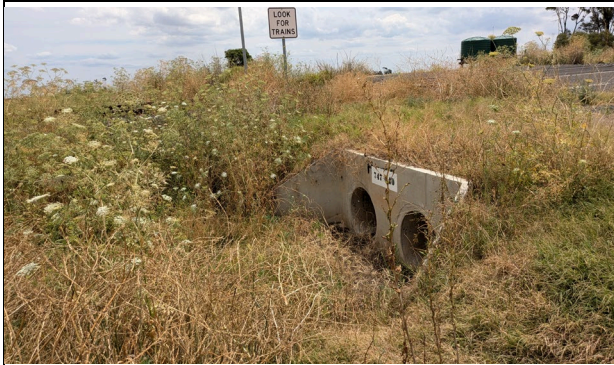
North of Boonery Park Rd – View north west at LX316 showing road culvert the discharge of which has resulted in erosion of rail maintenance access road materials to the Pearlman Property.
