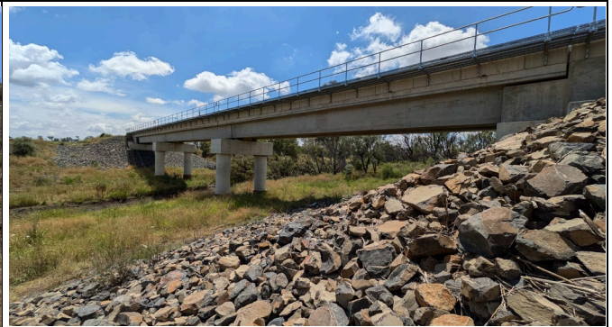
Croppa Creek bridge – View north across Croppa Creek showing area well vegetated.
