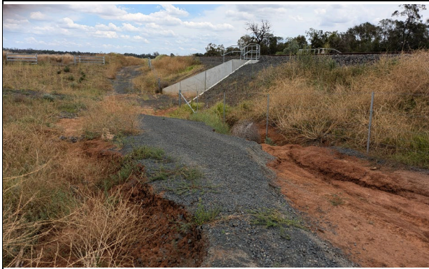
North of Boonery Park Rd - 745.879 significant scour of track access road rendering it inaccessible / unusable.
