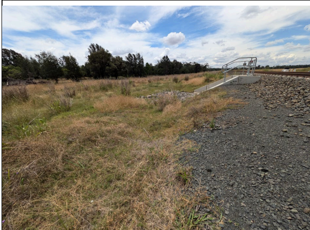
North of Boonery Park Rd – View north of 745.430 scour area within Pearlman Property with suspect mound blocking downstream flow on the left.
