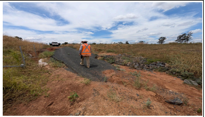
North of Boonery Park Rd - 745.879 scour of track access road showing failed erosion controls on the right.
