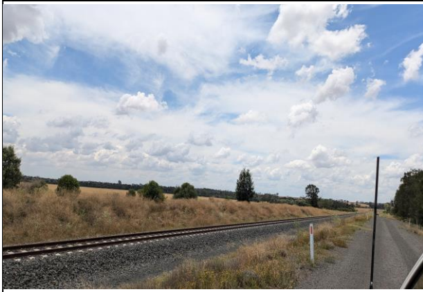
North of Boonery Park Rd, North Star – View north with new berms along alignment well vegetated
