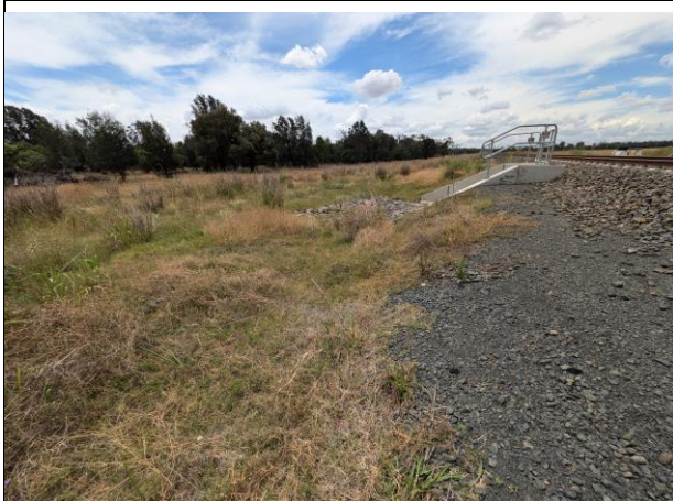
North of Boonery Park Rd – View north of 745.430 scour area within Pearlman Property with suspect mound blocking downstream flow on the left
