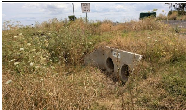
North of Boonery Park Rd – View north west at LX316 showing road culvert the discharge of which has resulted in erosion of rail maintenance access road materials to the Pearlman Property
