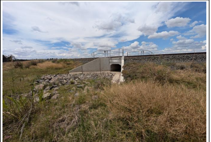
North of Boonery Park Rd – View northeast of 745.430 scour area within Pearlman Property with same suspect mound seen on the right diverting flow to culvert
