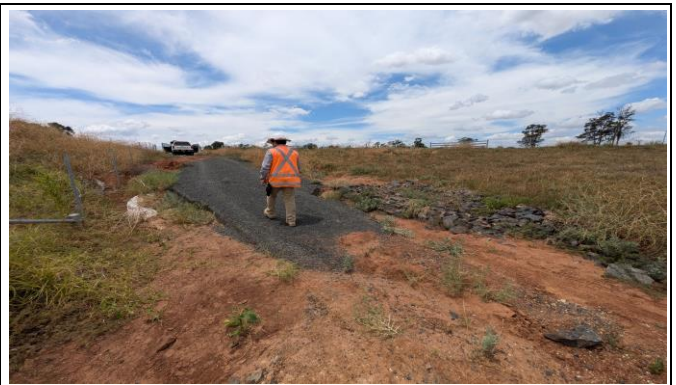
North of Boonery Park Rd - 745.879 scour of track access road showing failed erosion controls on the right
