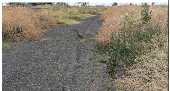
North of Boonery Park Rd – View north at LX316 showing erosion of the rail maintenance access road along Pearlman property, downstream of the road culvert, after some repairs
