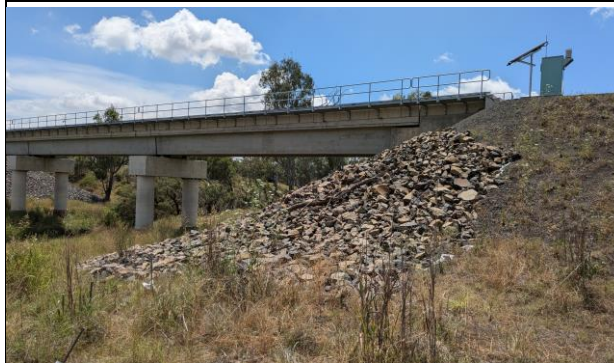
Croppa Creek bridge – View northwest across Croppa Creek with flood monitor visible on the right.
