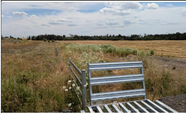
North of Boonery Park Rd -LX3165 area of scour within Pearlman Property
