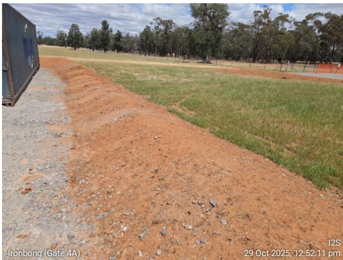
Figure 1: MAF Ironbong Rd (CH9380) – berm to stabilise
