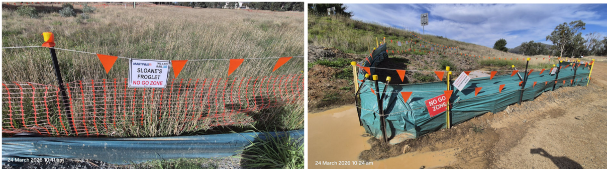
Figure 7. Billy Hughes – Sloane Frog habitat protection (24/03/26 ER inspection)
