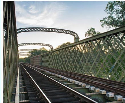
Figure 25. Standard and broad gauge lines on the Murry River Rail Bridge. Source: Inland Rail.
