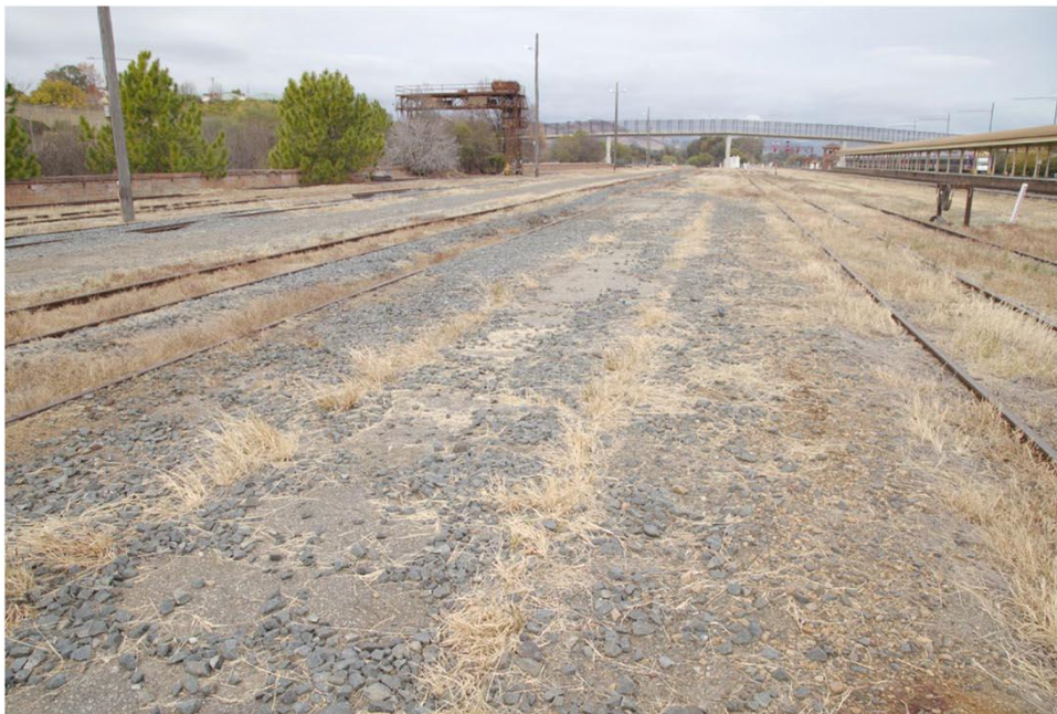
Figure 46. View of Track 3 facing south, showing the rails covered with ballast and grass. Source: Extent Heritage.
