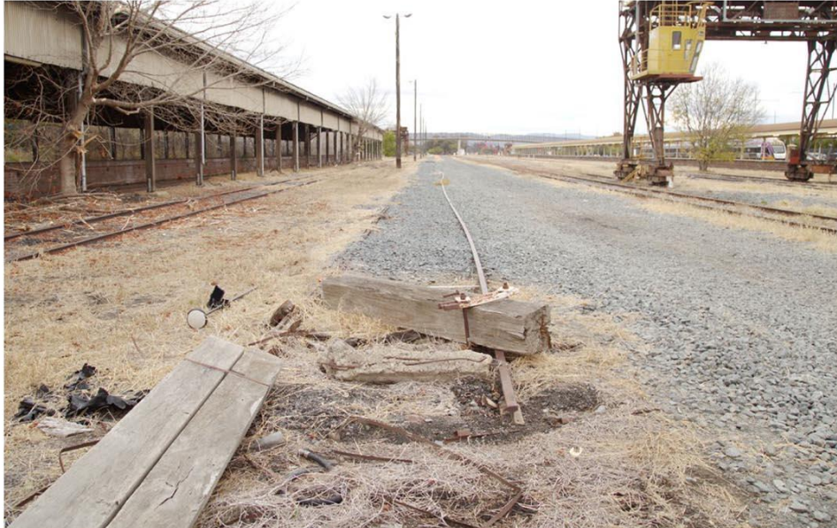
Figure 40. Northern end of Track 5 showing debris piled on top of track. Source: Extent Heritage.
