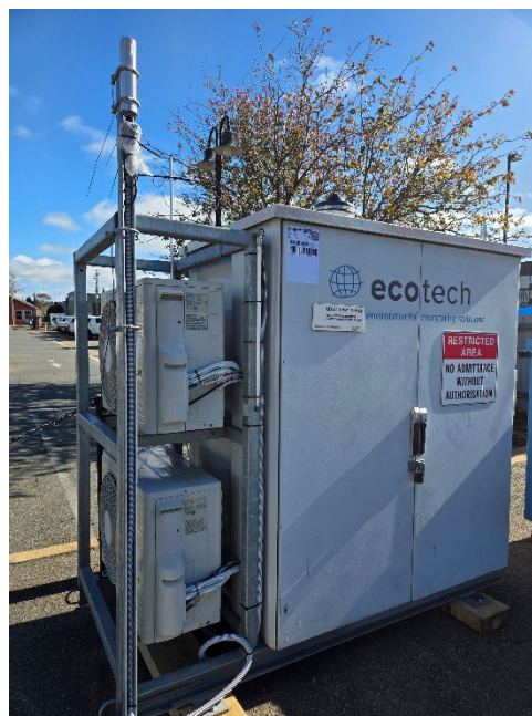
Air monitoring unit
