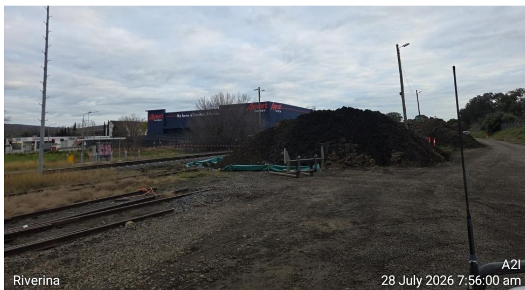
Figure 1. Riverina – Spoil stockpile to be protected or removed (28/07/26)
