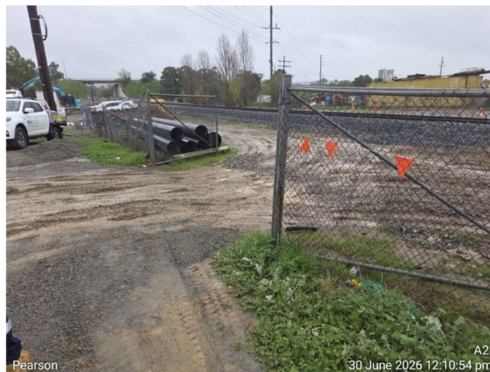
Figure 1. Wagga Wagga Pearson – Insufficient exit control at gate (30/06/26)
