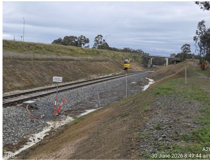
Figure 4. Billy Hughes Bridge - Unprotected batters (30/06/26)
