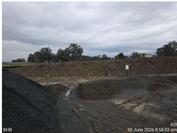
Figure 5. Billy Hughes – ASSTA bund breached, stockpile neutralised, sediment traps located downslope (30/06/26)
