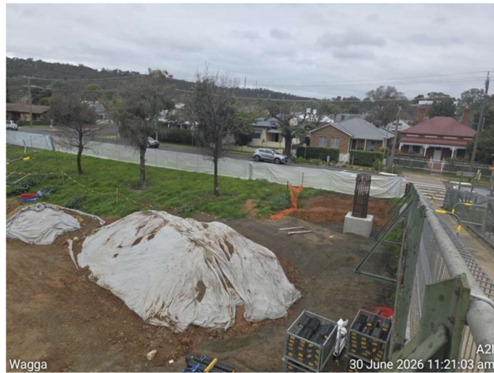
Figure 6. Wagga Wagga Mothers FB – CIZ Flagging damaged (30/06/26)
