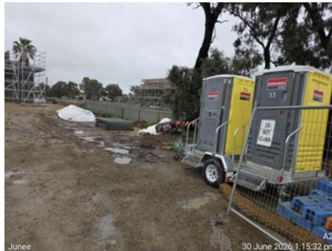
Figure 2. Kemp St Eastern side Gate 6 – geofabric and other materials under tree dripline (30/06/26)
