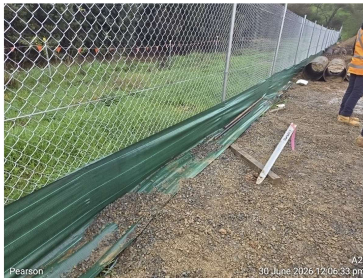
Figure 7. Wagga Wagga Pearson – Toe of sediment fence unsecured (30/06/26)
