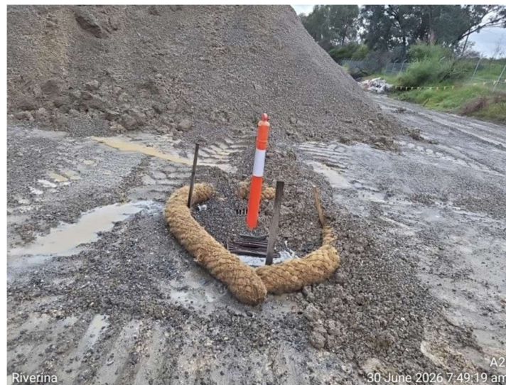
Figure 3. Riverina, Albury – Damaged inlet control (30/06/26)
