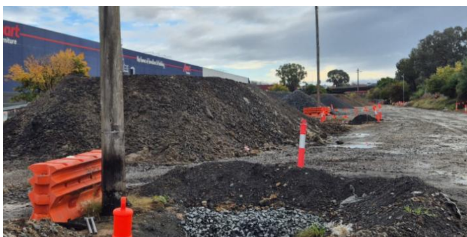
Figure 3. Riverina, Albury – unprotected stockpiles (19/05/26)
