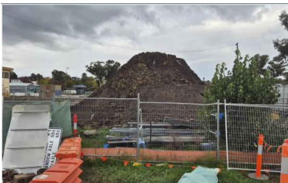
Figure 8. Kemp Street – unprotected stockpile (19/05/26)
