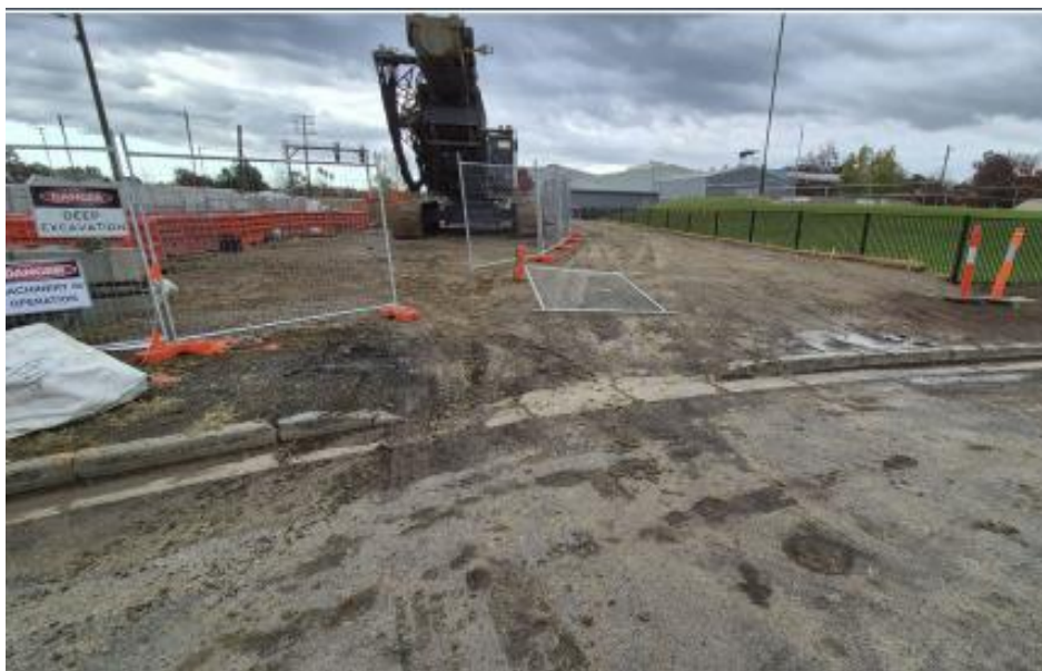
Figure 7. Junee – construction access with insufficient controls (19/05/26)
