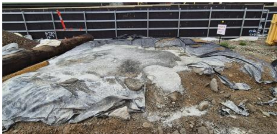
Figure 4. Edmonston Street – concrete washout requiring maintenance (19/05/26)
