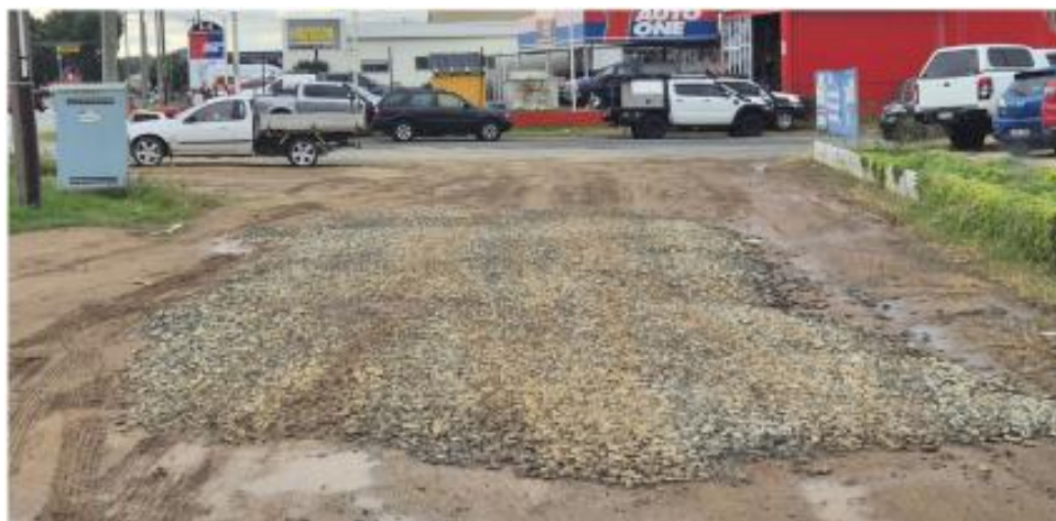
Figure 5. Pearson & Cheshire St – construction access with insufficient controls (19/05/26)
