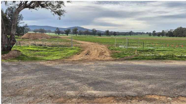
Figure 1 Ironbong Road Gate 4.1 – unstabilised construction access (17/06/26)
