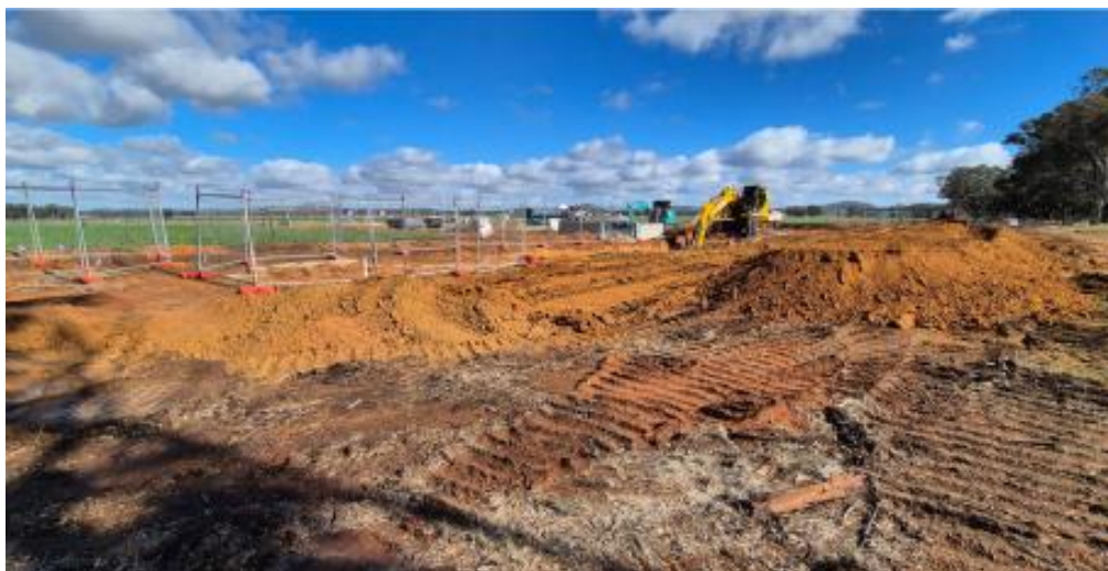
Figure 4. Burley Griffin Way –works requiring additional erosion and sediment control measures (20/05/26)
