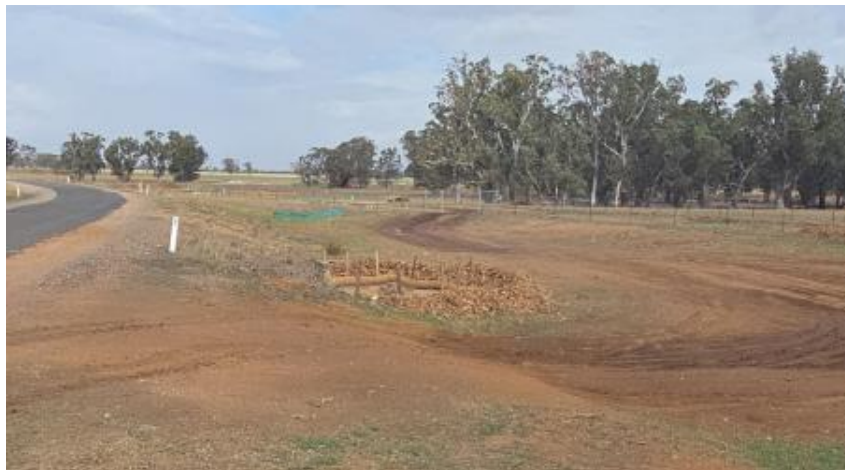
Figure 1 Ironbong Road – unstabilised construction access (03/05/26)
