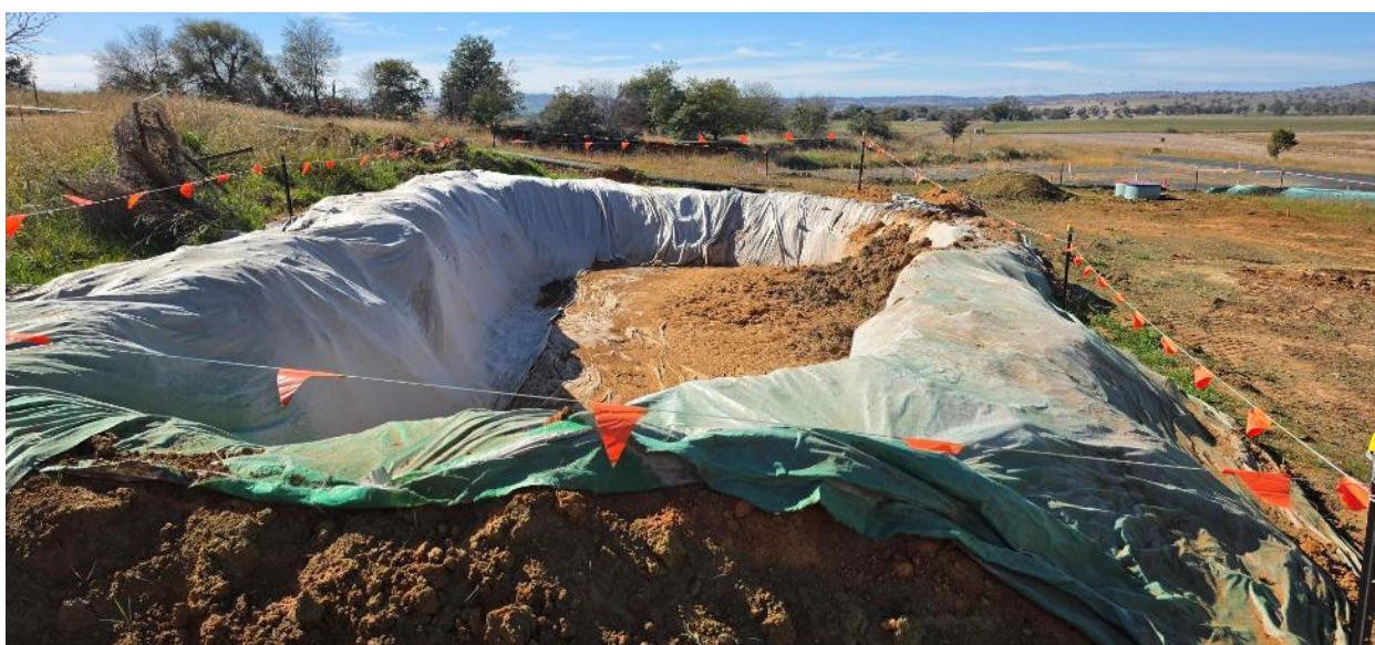
Turkey's nest installed for water storage and reuse.
