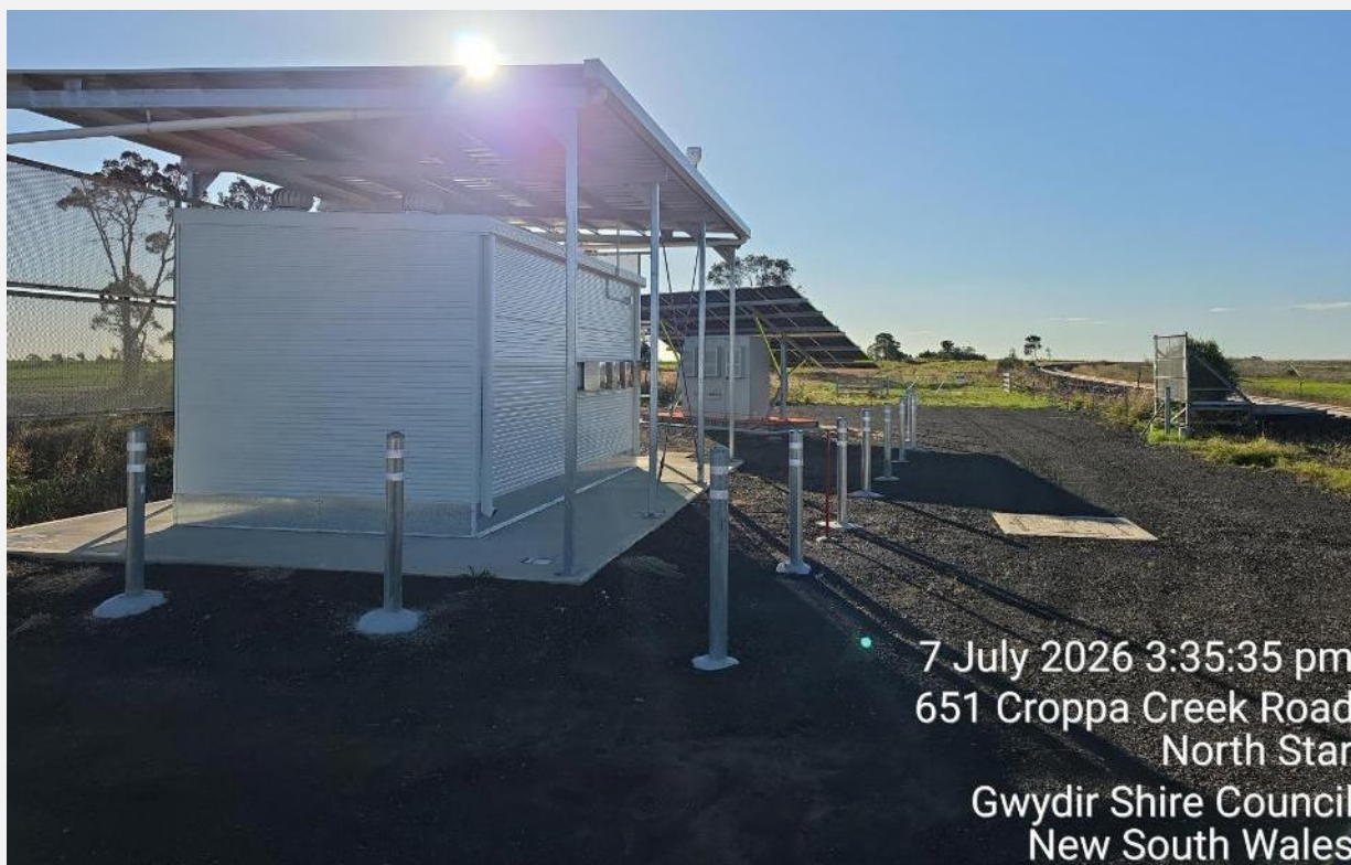
Solar-powered level crossing signal infrastructure installed at LX 3166.
