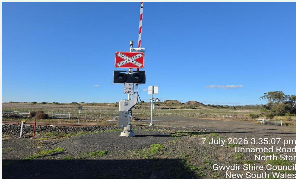
Solar-powered level crossing signal infrastructure installed at LX 3166.
