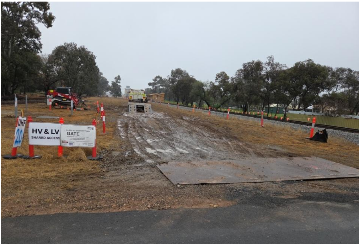
Figure 3. Gate 14 Stockinbingal - additional access stabilisation to be undertaken (26/08/26)
