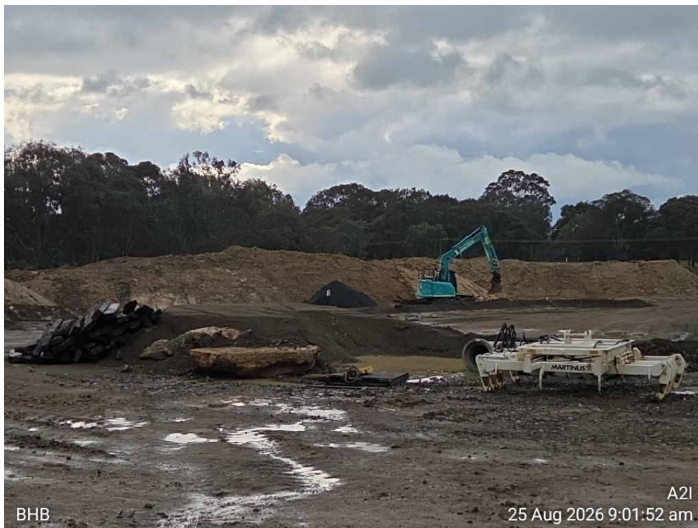
Figure 2. Billy Hughes Bridge – Spoil stockpile to be protected or removed (25/08/26)
