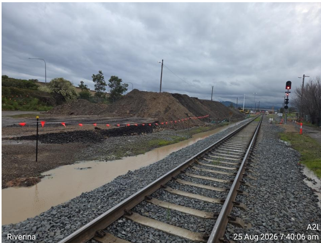
Figure 1. Riverina – Spoil stockpile to be protected or removed (25/08/26)
